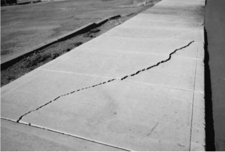
Figure 23.1 A substantial crack in a sidewalk with low frequency of pedestrian traffic.
