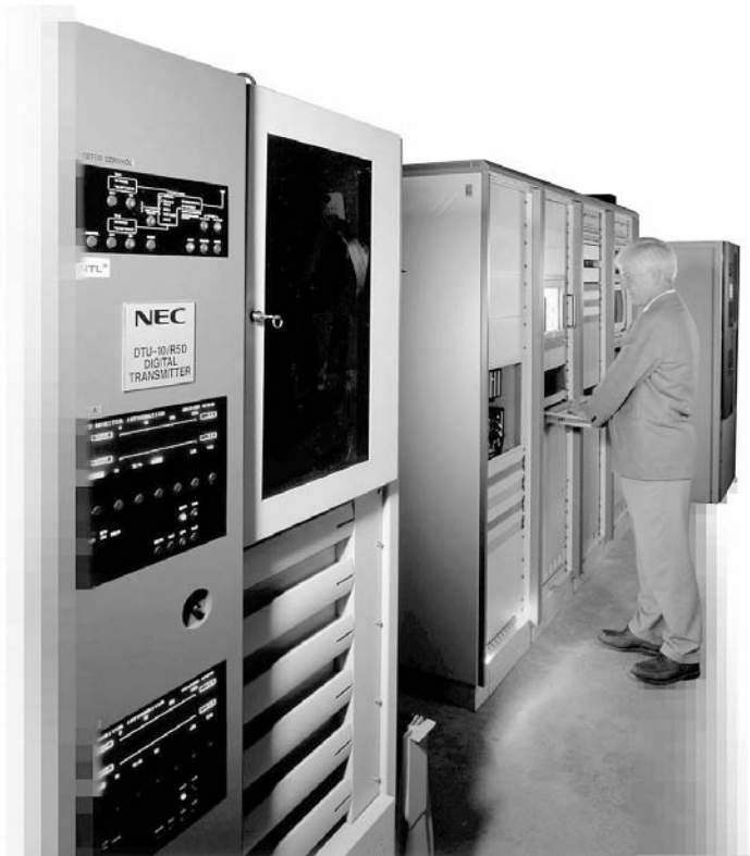
Figure 2.8 TV transmitters – digital (Courtesy NTL)
