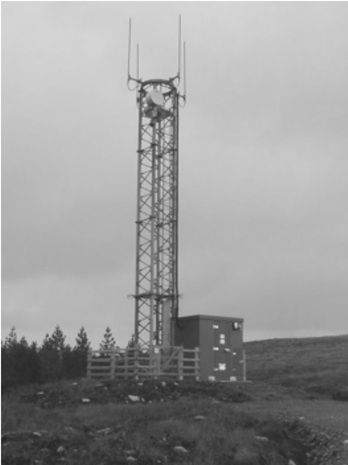
Figure 6.13 Tower mounted colinear antennas (Courtesy of BT)
