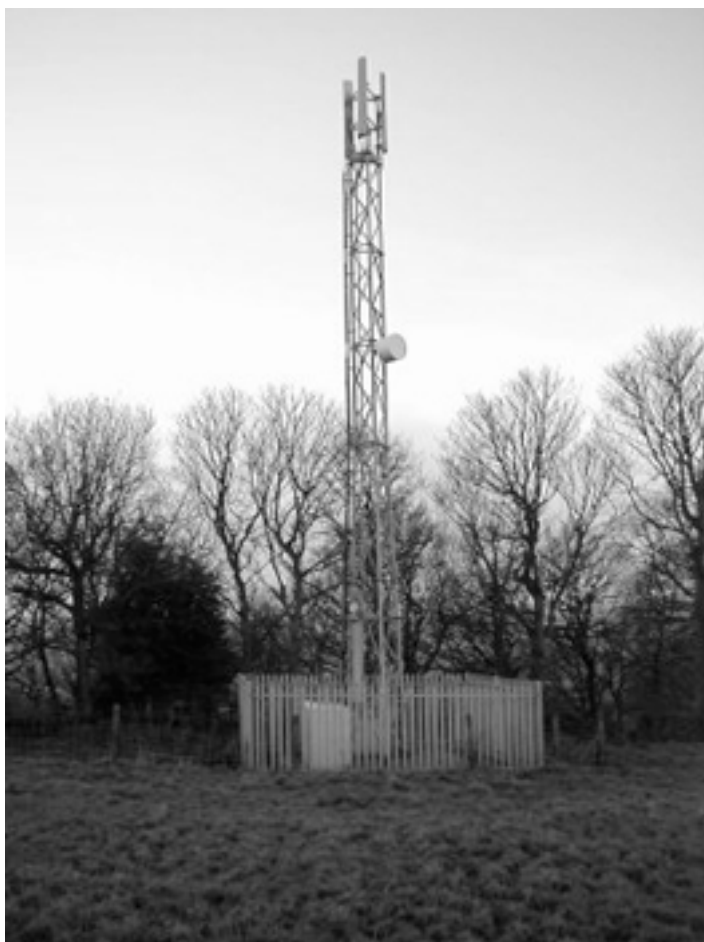
Figure 6.12 Tower-mounted sector antennas (Courtesy of BT)
