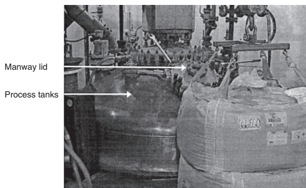
FIGURE 12 Process tank with sealed manway.
