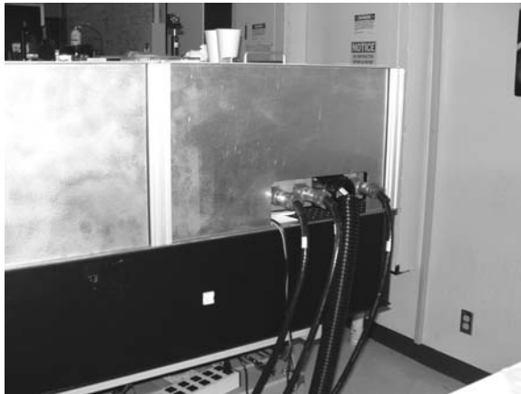
FIGURE 14.8 Cables out of enclosure.
