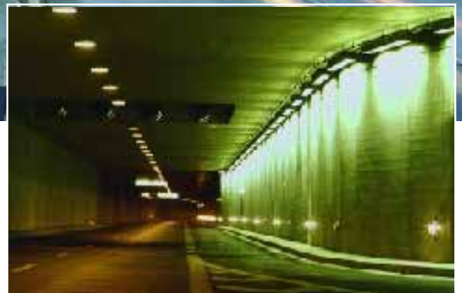
The lighting inside a tunnel at night should be brighter than the street lighting outside. This counteracts any oppressive sensation of confinement within the tunnel. 80
