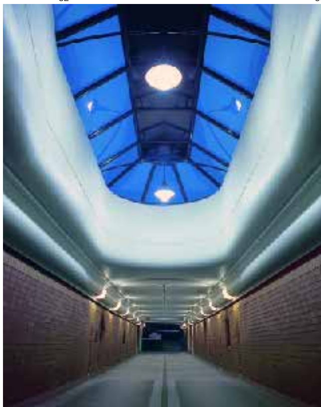
Safe conduct: the lighting accompanies pedestrians from one end of the underpass to the other.
