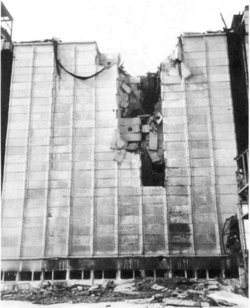
Figure 4-11 The concrete silo complex in Tomylovo, Knibyshev region, Russia that was damaged by a series of smoldering gas explosions in the silo cells. (Courtesy of A. Borisov and B. Gelfand, Moscow, Russia).
