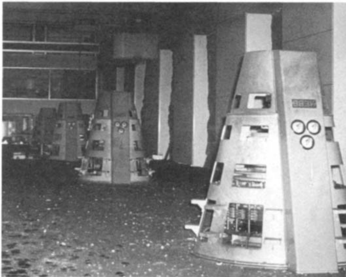
Figure 3-13 Photo of debris after the oil spray/mist explosion in the main hall of the underground hydroelectric power station at Tonstad, Sirdal, Norway, illustrated in Figure 3-10. The conical cabinets of the control instruments are seen clearly.
