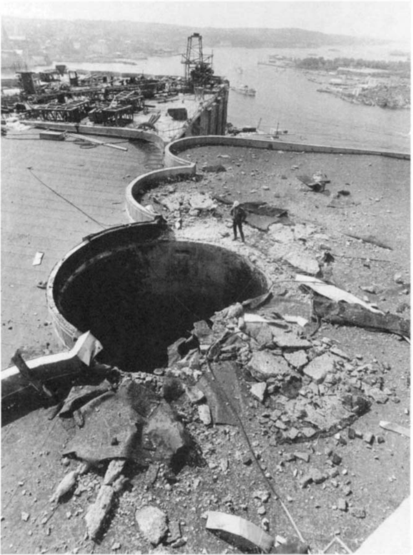
Figure 5-42 Damaged silo roof after the wheat grain dust explosion in Stavanger in June 1970. From Eckhoff (2003).
