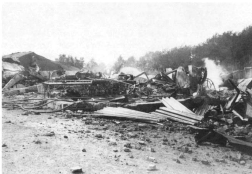
Figure 5–48 Scene of total demolition after aluminum dust explosion in the premix plant of a slurry explosives factory at Gullaug, Norway, in August 1973. From Eckhoff (2003).
