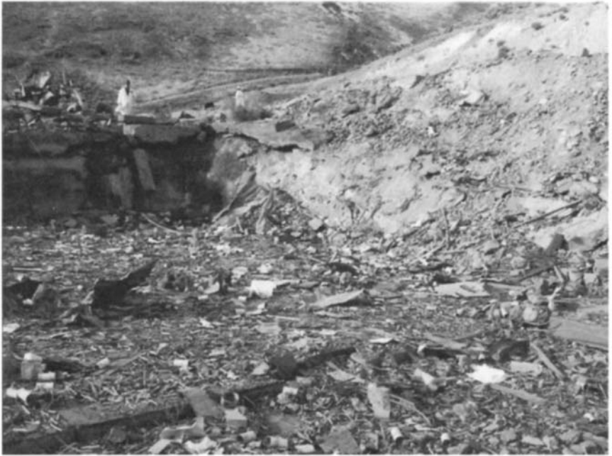
Figure 6–10 Remains of Booster Room 2 of the Sierra Chemical Company Kean Canyon plant east of Reno near Mustang, Nevada, USA, after explosives mix explosion in 1998. From CSB (1998).
