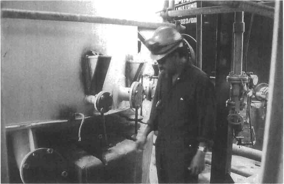
FIGURE 3-3 Tank bottom is bulged during a hydrotest.
