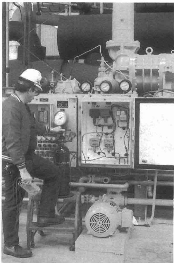
FIGURE 9-22 Prooftesting a high-pressure switch on a refrigeration unit.
