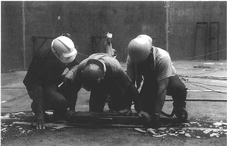
FIGURE 9-13 Inspectors using a vacuum box and soapy water to check for leaks in welds on the floor of a low-pressure tank.
