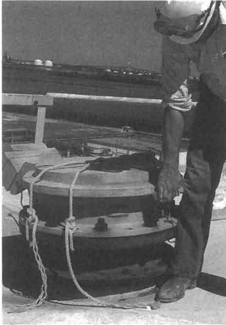
FIGURE 6-10 Hinged vent lid improperly tied to cope with anticipated high winds and to prevent intrusion of rain.
