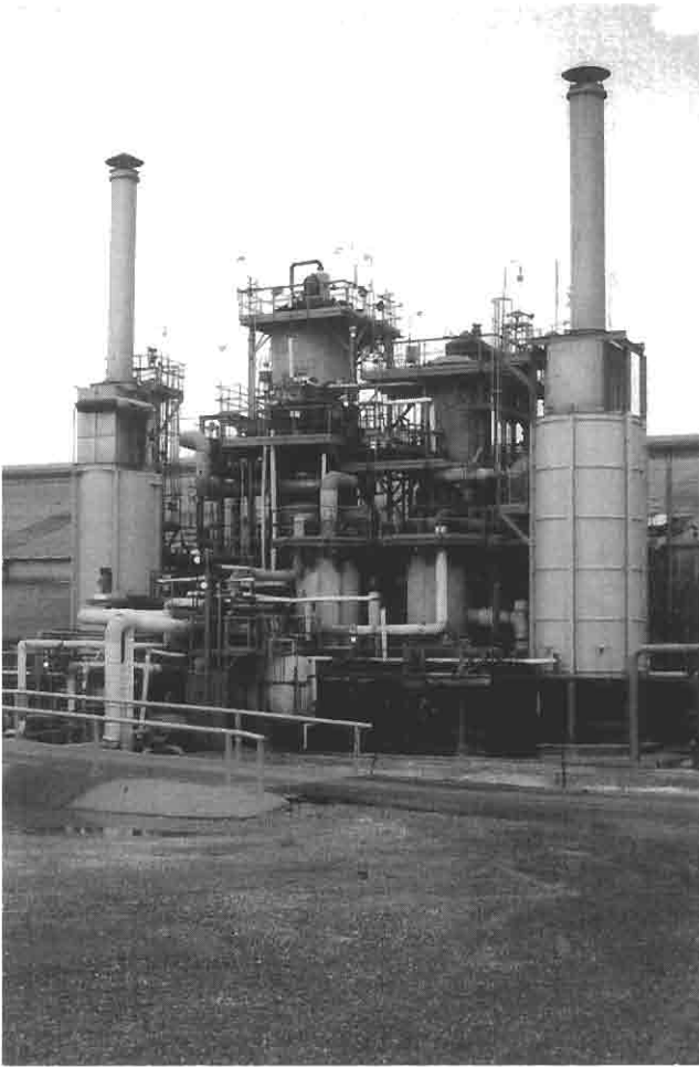
FIGURE 6-5 Well-maintained unit is troubled by a leak.
