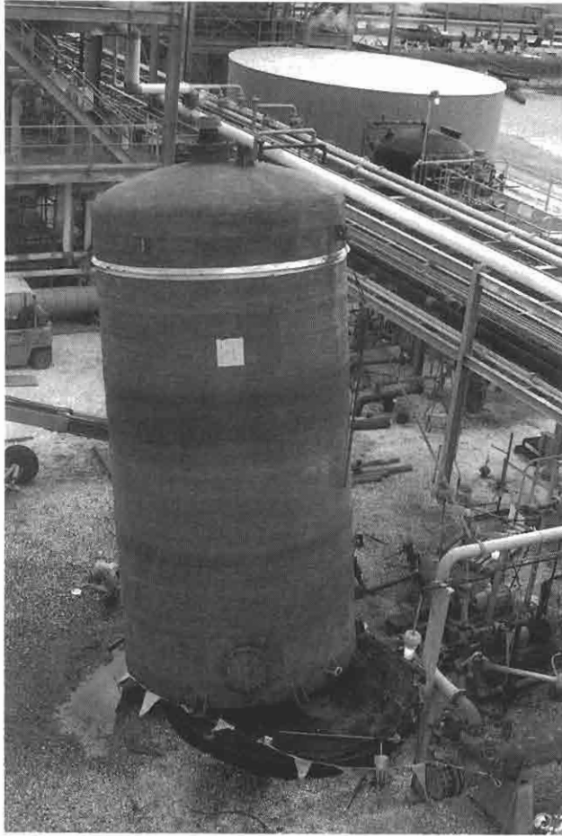
FIGURE 5-12 An aerial view of the tank failure.
