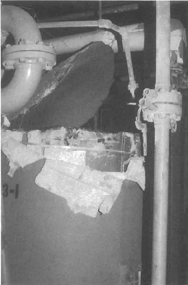
FIGURE 2-22 Close-up of the failed air dryer.
