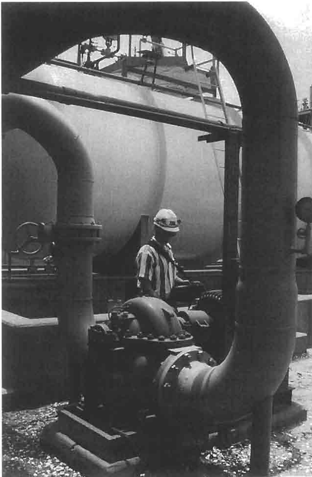
FIGURE 9-2 A vibration technician taking readings on a cooling water pump.
