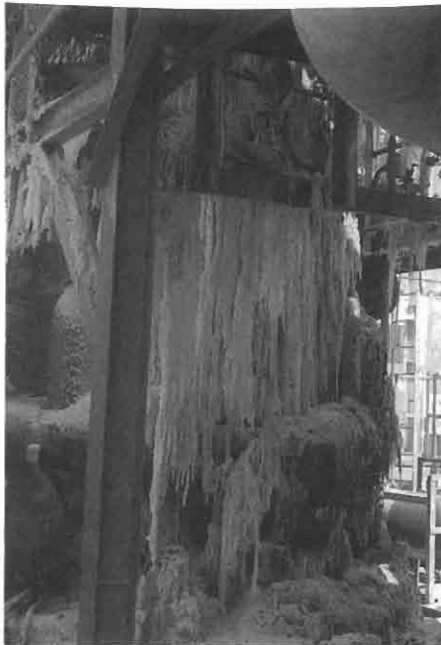
FIGURE 6-7 Icicles are formed from leaking caustic soda that dripped from an evaporator flange.
