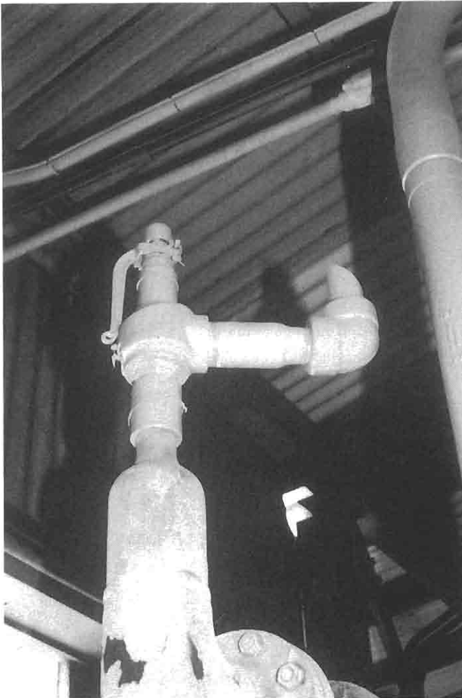
FIGURE 6-13 A threaded SRV valve reinstalled with a reduced discharge piping arrangement.
