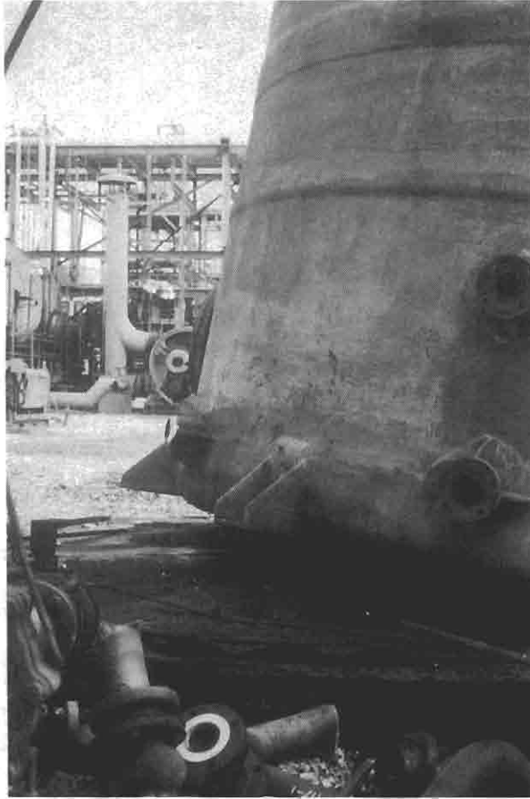
FIGURE 5-13 A close-up of the failed tank base.
