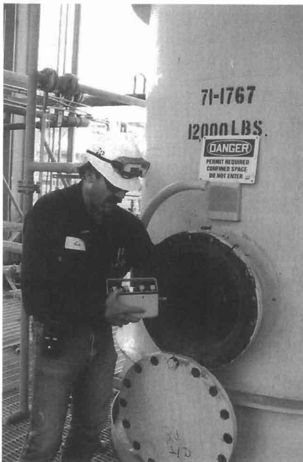
FIGURE 9-8 An operations foreman checks for blinding and samples the vessel's atmosphere before tank entry.
