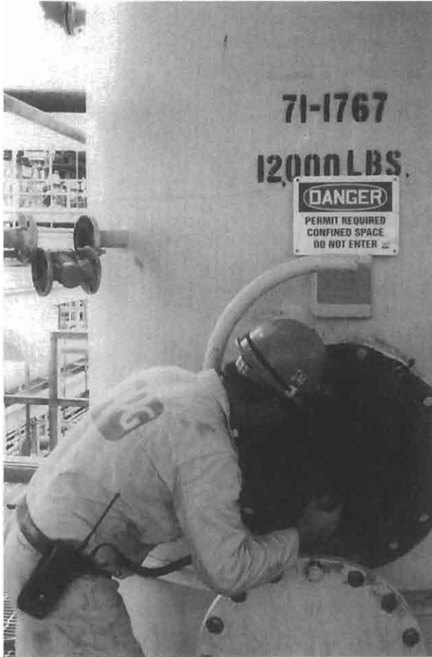
FIGURE 9-9 A pressure vessel inspector making an initial assessment of the vessel to determine any special inspection needs such as ladders, scaffolding, or extra lighting.
