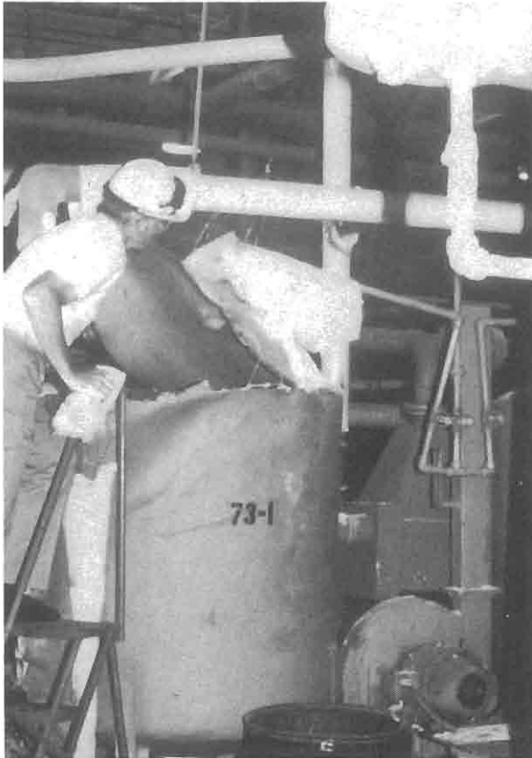
FIGURE 2-21 Employee examines the air dryer failure.
