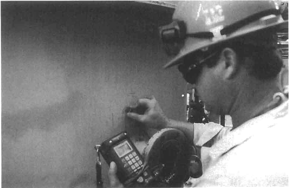
FIGURE 9-11 An inspector verifying wall thickness on a vessel near a nozzle that had experienced metal loss.
