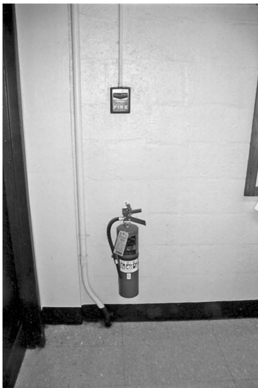
FIGURE 25.13 Fire extinguisher in close proximity to the alarm box.
