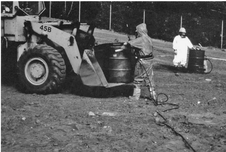
FIGURE 23.7 Workers must be fully protected when dealing with hazardous waste.
