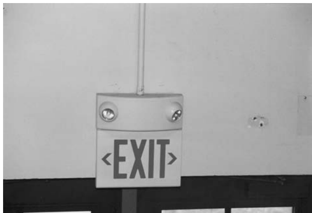
FIGURE 25.11 Example of an exit sign.
